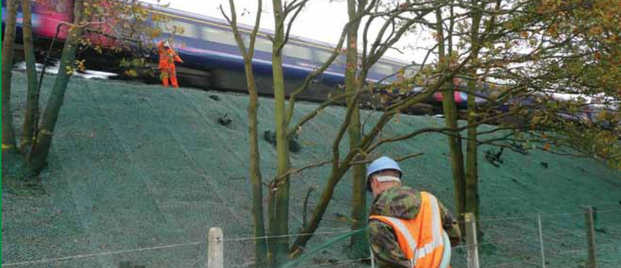
Spraying HydraCX™ through rock netting on a soil nailed embankment for a rail project, UK.
