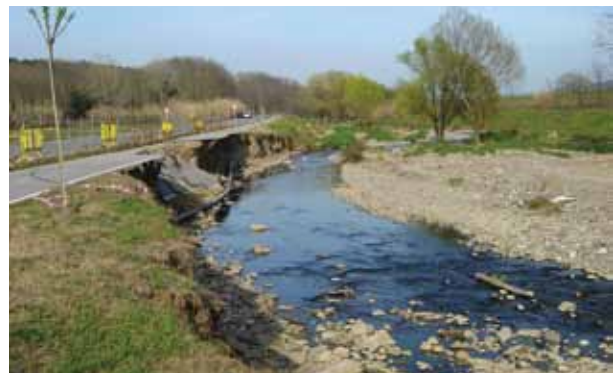
Erosion has undermined this cycle path and now threatens the safety of the adjacent road.
